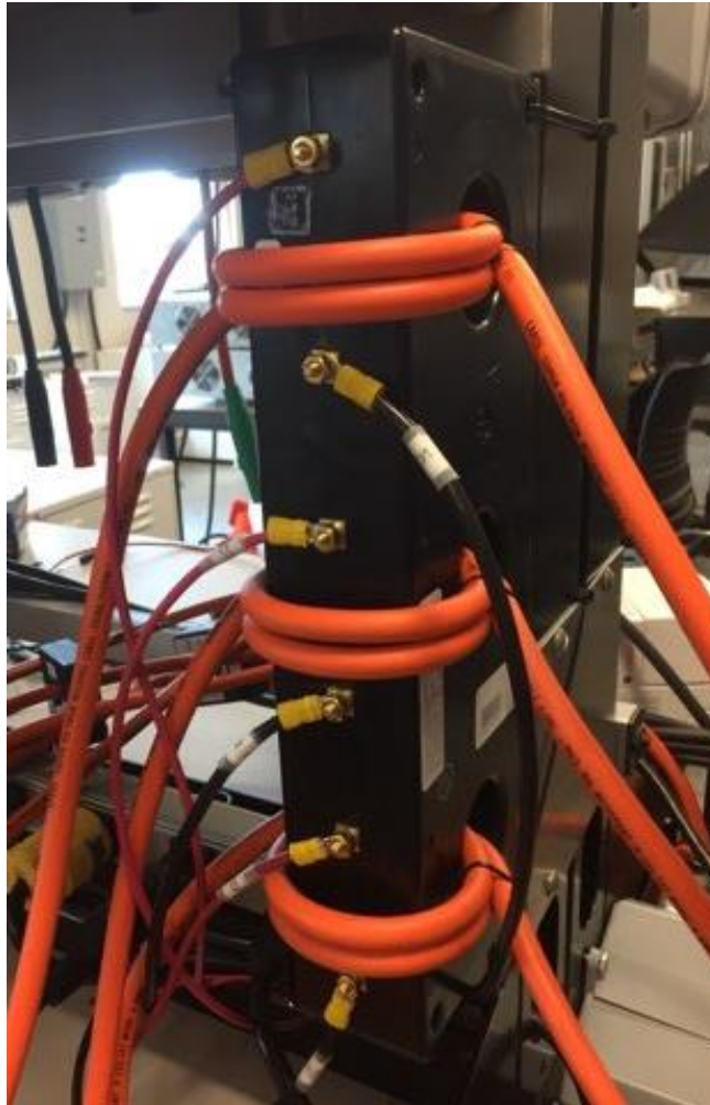
Figure 7: GE 3P40-101 Current Transformer
