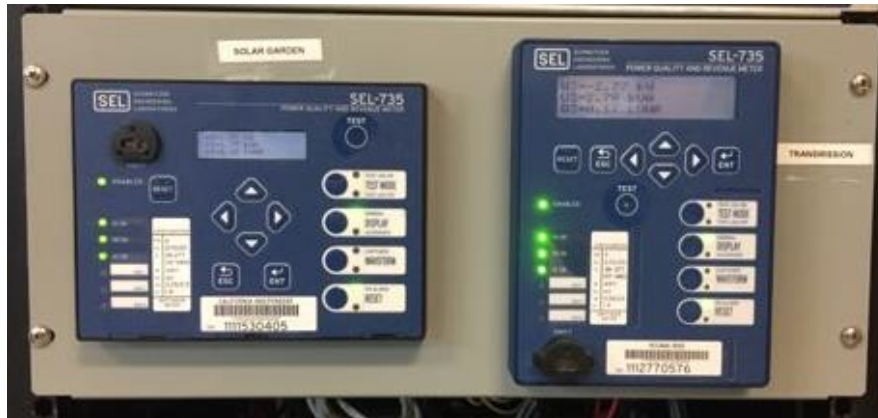
Figure 6: SEL-735 Power Meters
