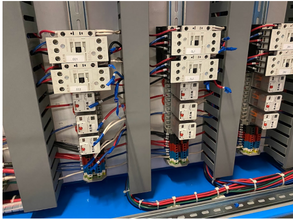
Figure 4: Loads taped off at the contactor level.
