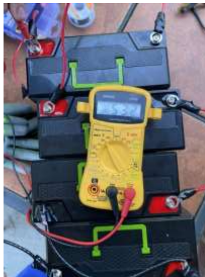
Figure 3: Voltage Reading (Series Batteries).
